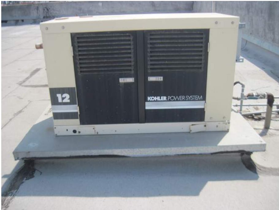
12. Emergency generator located on Food 4 Less rooftop.
