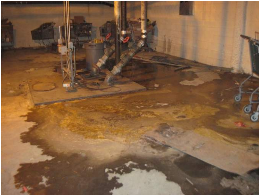
14. Sump and pump equipment in parking garage of Food 4 Less (note grease on surface of water).
