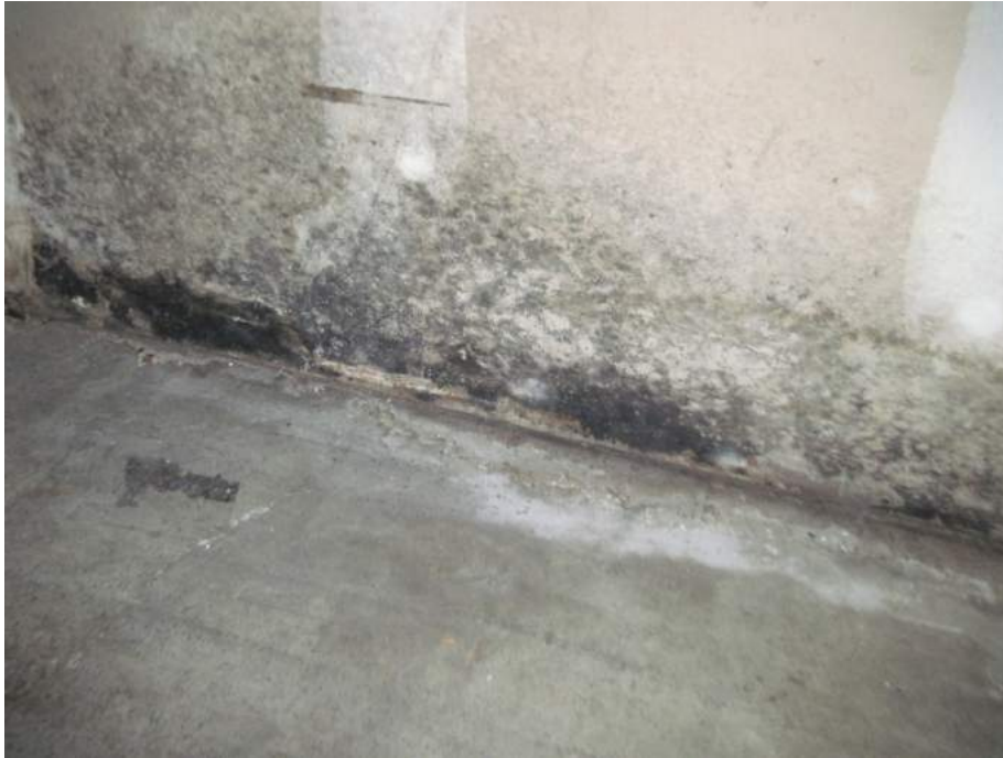
17. View of suspect mold growth in basement electrical room of Food 4 Less.
