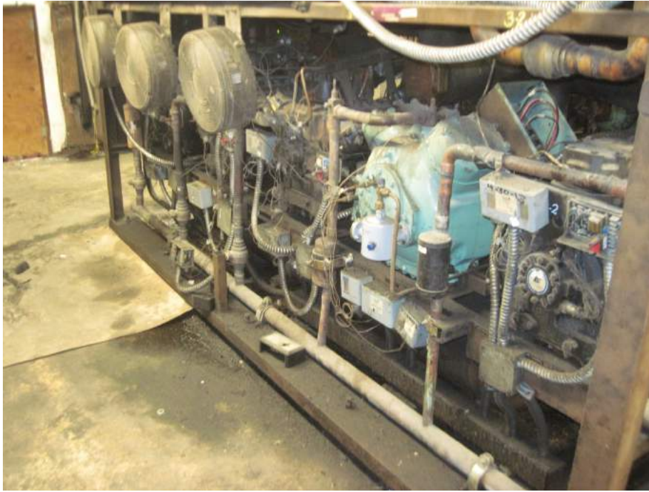
9. Oil staining beneath compressor in Food 4 Less mezzanine.
