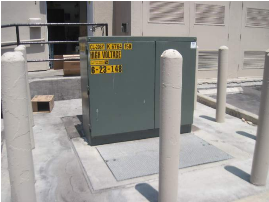
18. Pad-mounted electrical transformer south of McDonald's.
