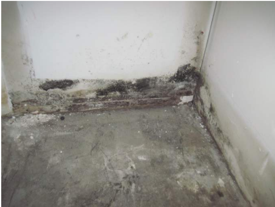
16. View of suspect mold growth in basement electrical room of ICDC.
