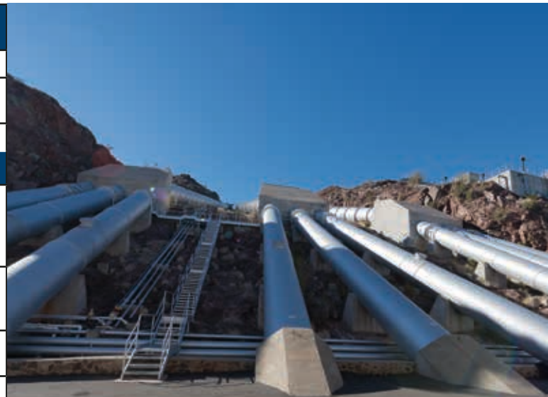
Delivery lines at Whitsett Intake Pumping Plant
