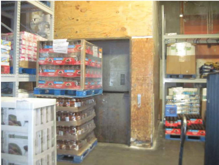
6. Out of service freight elevator in Food 4 Less.
