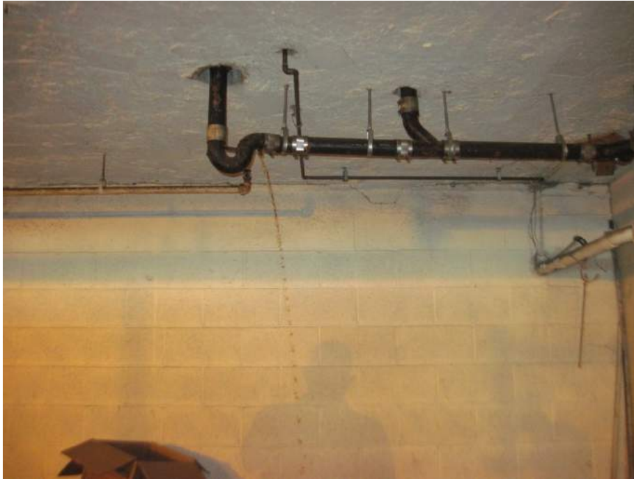
15. Water leaking from above basement level garage into sump area.
