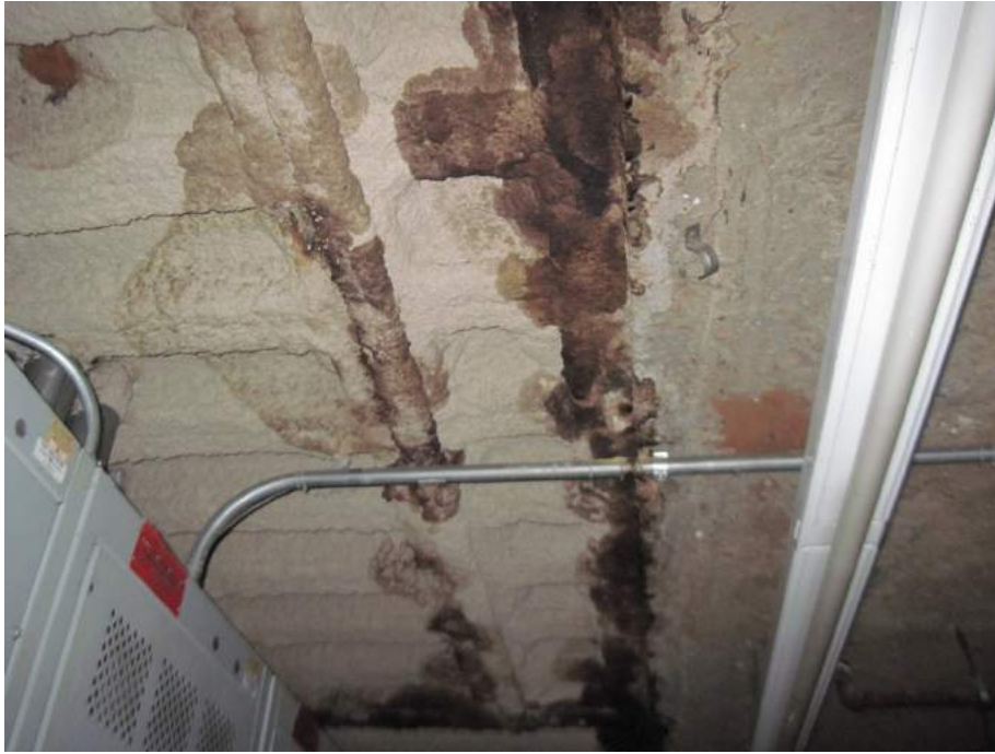
19. Water-damaged fireproofing in basement electrical room of Food 4 Less.
